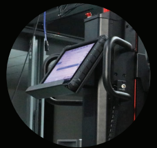
Consolidated Power Supply
